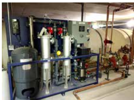
UV System Installation
