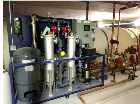
UV System Installation
